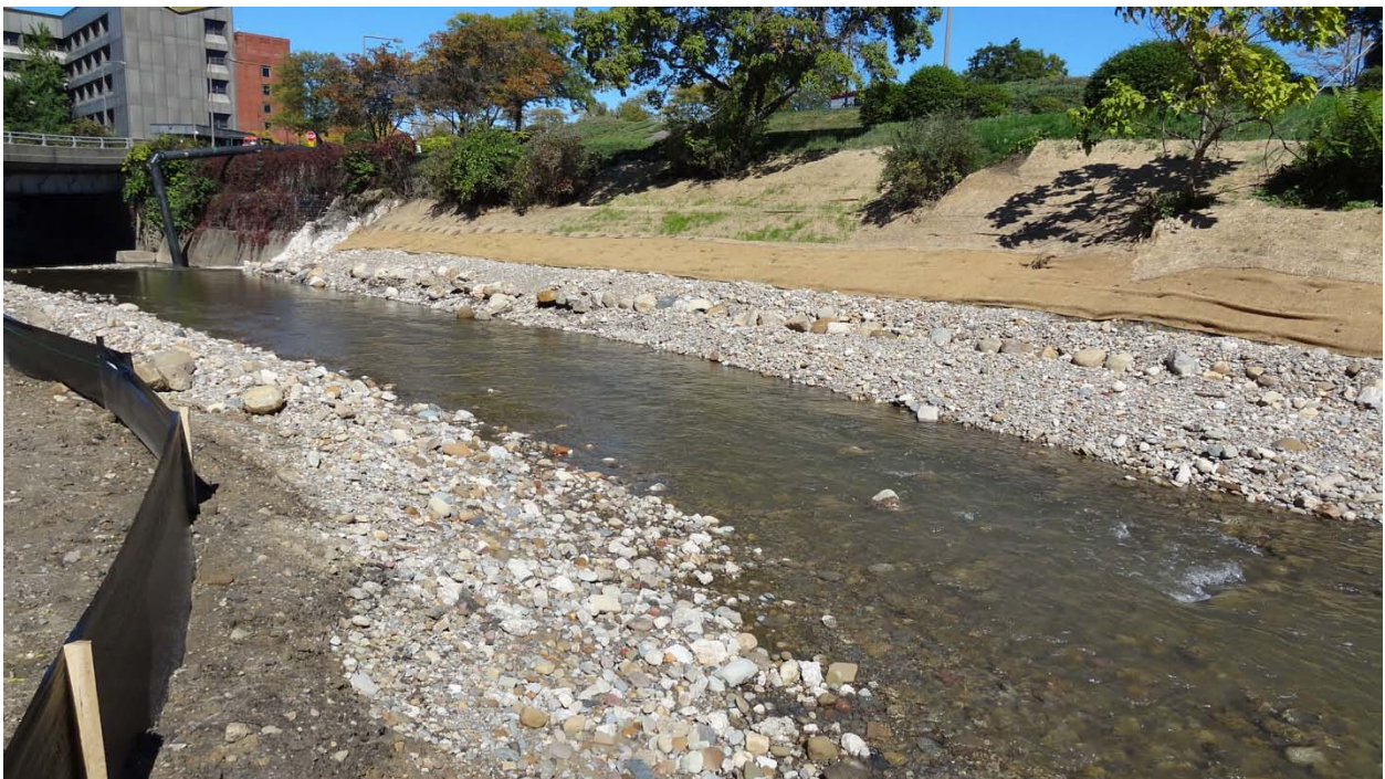
September 24, 2012 Looking downstream from midpoint of dam and Kelly Ave. This is the former dam impoundment area.
