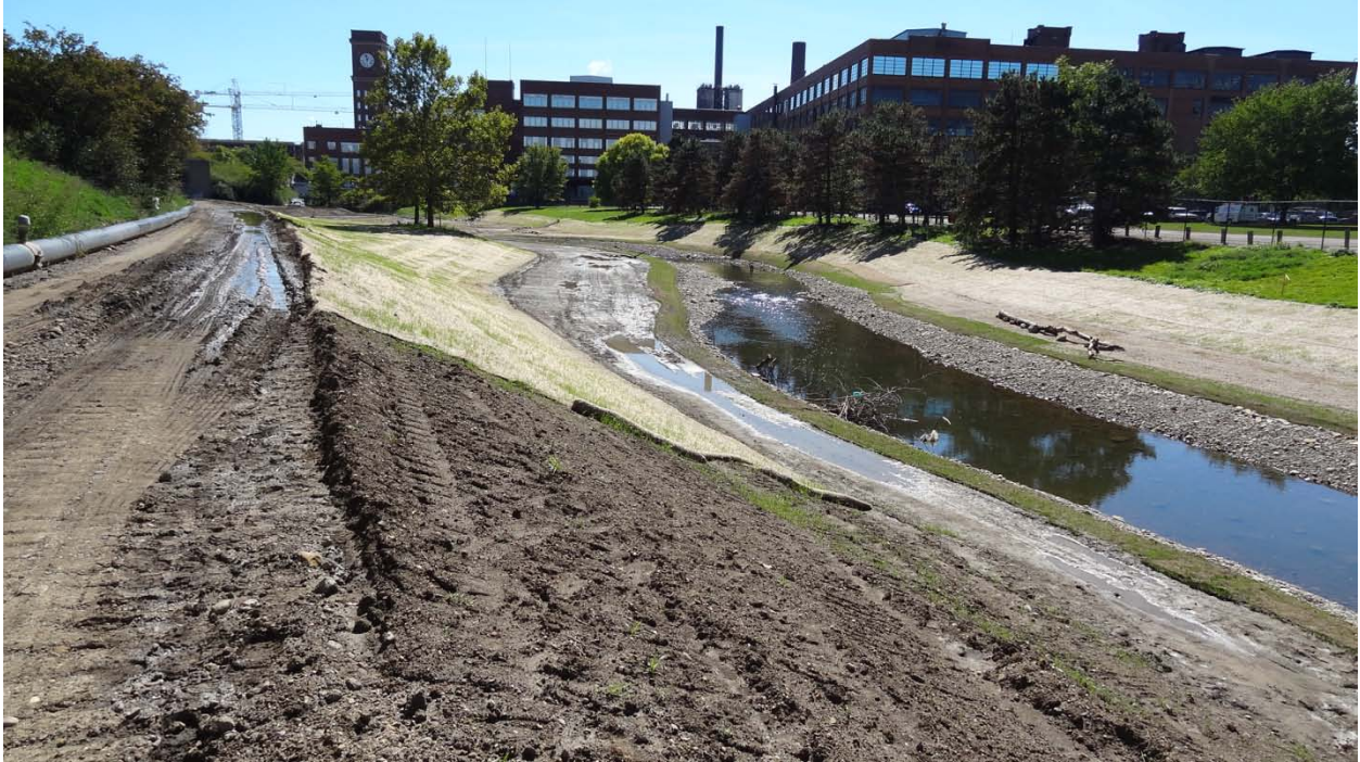
September 24, 2012 – Looking upstream from I-76 toward Martha Ave. Seeding and sod is establishing on banks.
