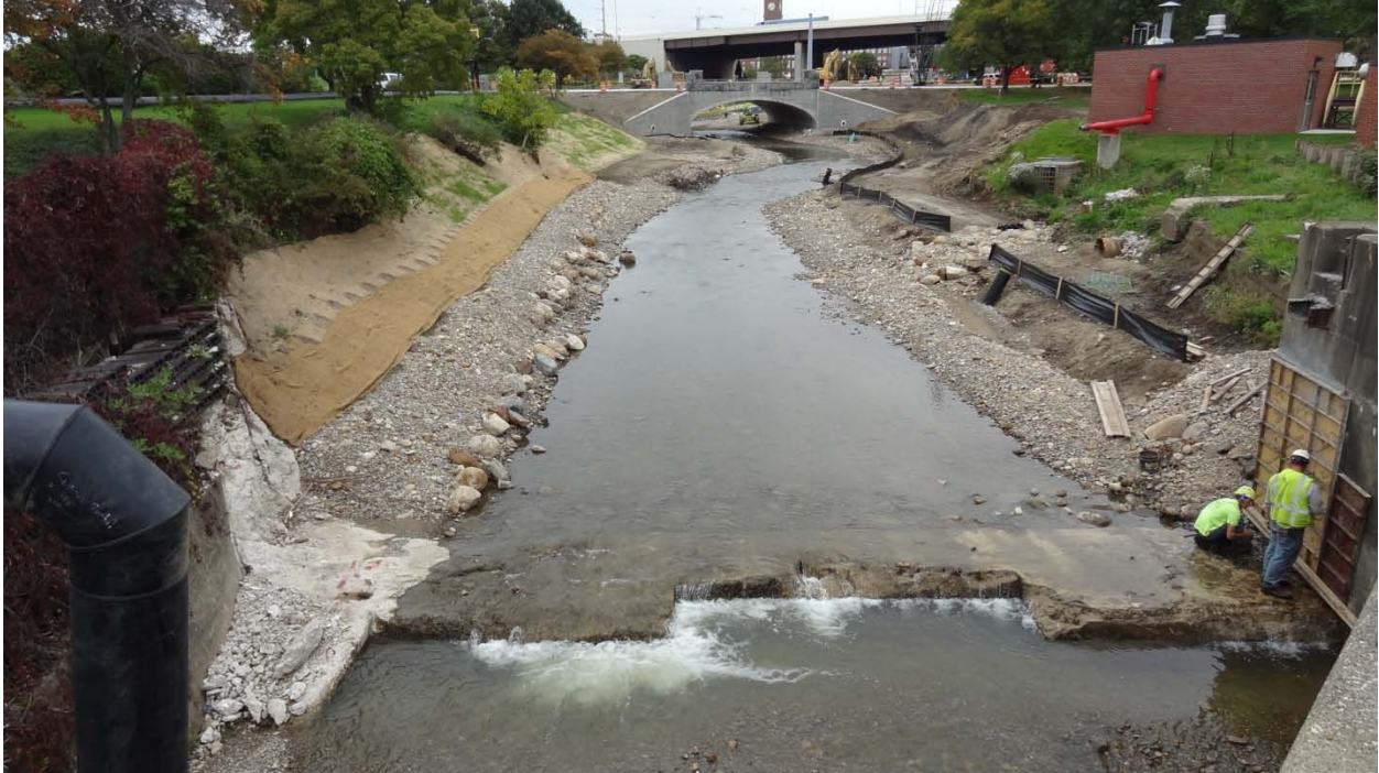
September 25, 2012 Looking upstream from former Kelly Ave bridge at lowered dam and replaced Kelly Ave bridge in background.
