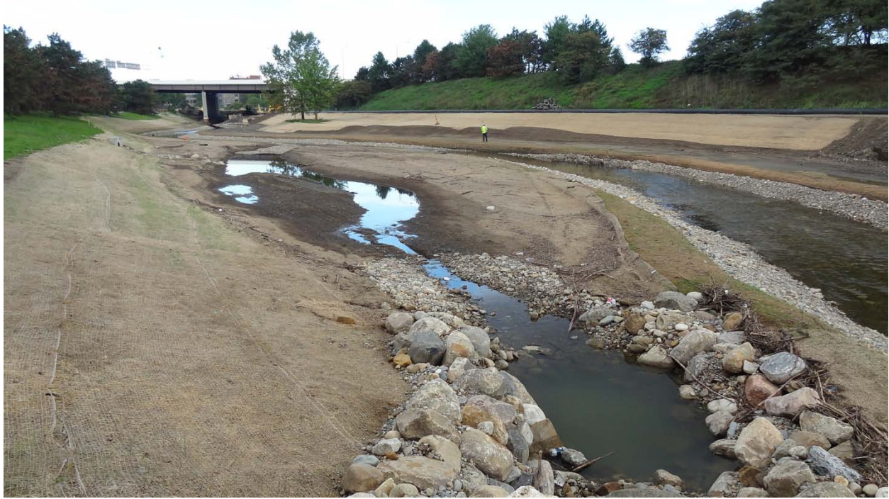
September 10, 2012 - From Martha Ave (Innovation Way) looking downstream. Little Cuyahoga River to right, wetland area to left.
